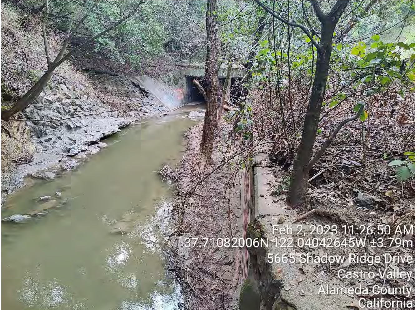
Photograph 4. Inlet of South Concrete Double Box Culvert and Retaining Wall, Looking South-Southwest
