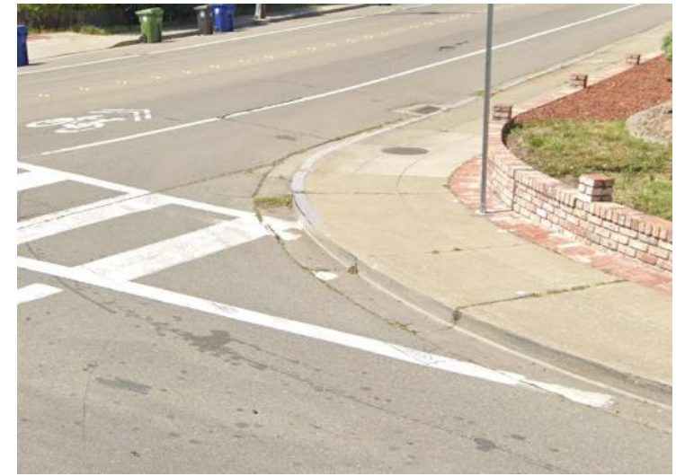
Curb return with no ramp
