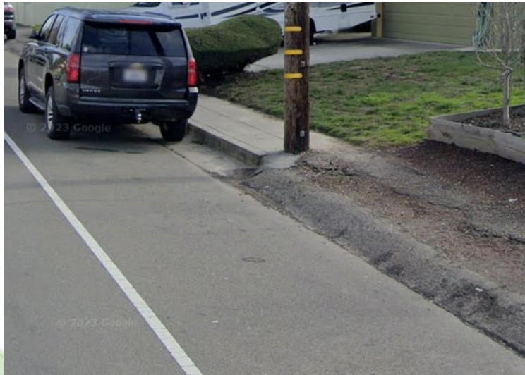
Gaps in sidewalk
