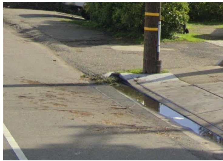
Ponding of water
