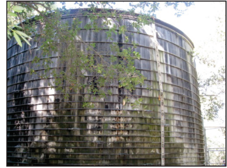
Figure 2-6 Upper Level Tank 1
