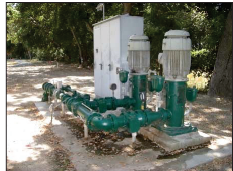
Figure 2-7 Valley Pump Station
